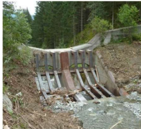
Large slot grill barrier for filtering (Leisnitzbach, Salzburg-Austria)
